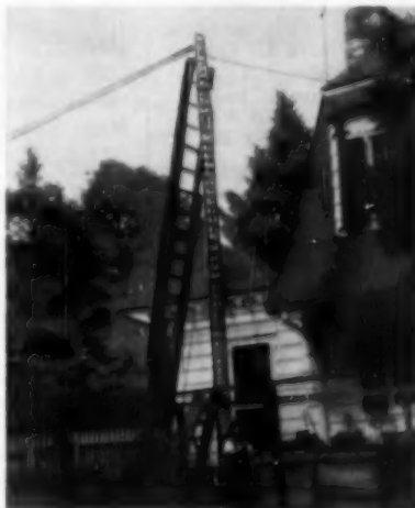
The collapsed tower, with its lower guy wires taut, is shown here just before the antenna rotator and antenna are mounted.
