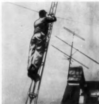
A final touch-up with aluminum spray is given the installation to cover worn spots caused by scraping during tower's erection.
