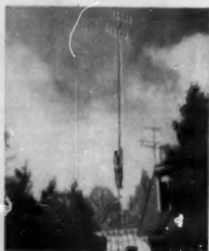
COVER PHOTO: A carefully installed antenna tower should be able to withstand winds of almost hurricane force. A few precautions taken at the time the tower is erected will pay off handsomely in the years to come. (Ektachrome by Jay Seymour)
